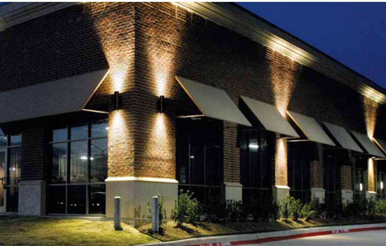
ALV uplight/downlight wall cylinders highlight brick texture while lighting the sidewalk.
